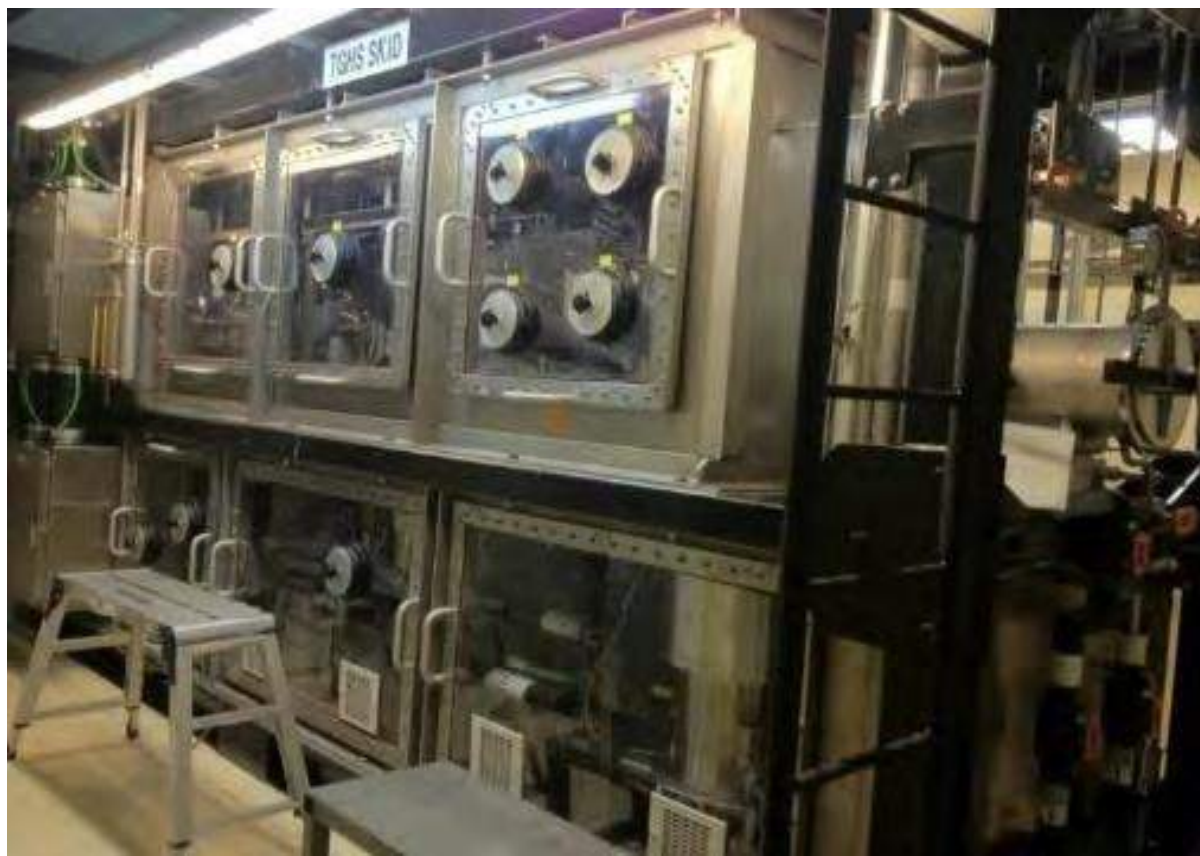
Figure 1.2.2.3.3 WTRF-Korea tritium gas handling and storage system
