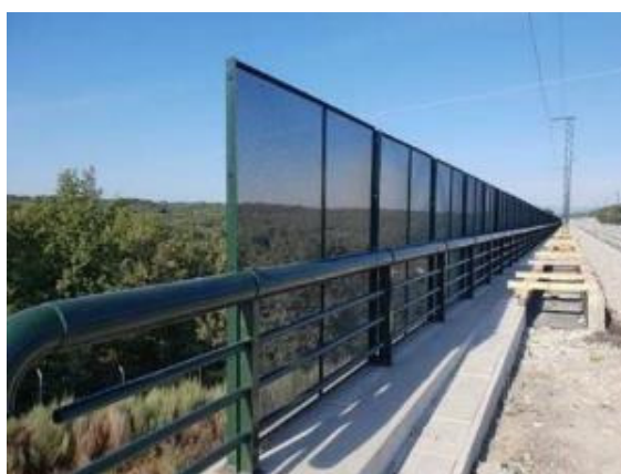
Figure no.2-5 Example of anti-collision panels
