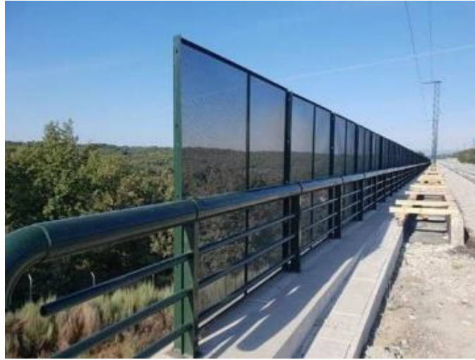
Figure no.7-2 Example of anti-collision panels (attention, the panels in the example are not 3m high)
