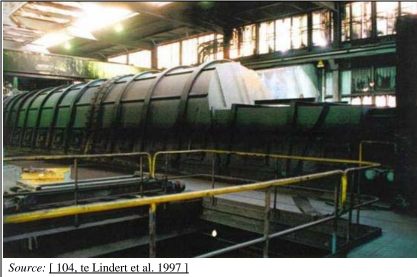
Figure 3.21: Covered sinter strand according to the EOS process
